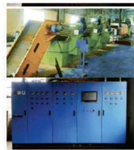
Continuous Hardening Furnace
